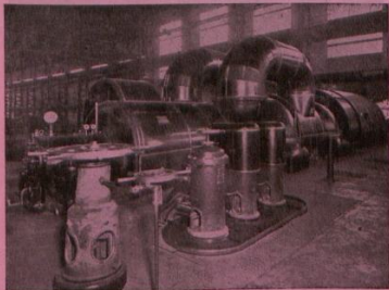
40,000 k.w. Turbo-Alternator installed at the Electricity Supply Commission Power Station at Congella.
