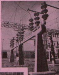
33 kV rotating type outdoor disconnects at Orlando Power Station, Johannesburg.
