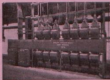
Low voltage metalclad H.R.C. fuse gear for control of boiler house auxiliaries.
