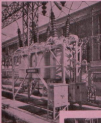
Type OKGJ 33 kV, 1,500 MVA outdoor type oil circuit breakers at Orlando Power Station, Johannesburg.
