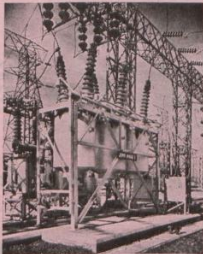
Type OKGJ 88 KV Outdoor type Oil Circuit Breaker, 1,500 MVA at Orlando Power Station.
