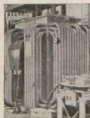
No. 446 a. Part of Scott connected bank supplying ovens in pottery works. Shown with the duplicate motors and pumps for pumping the oil through the coolers. Details of the transformers are as follows: 360 kVA., H.V. 6,600 volts, L.V. 60 volts 3,850 amps. Weight of transformer is 5 tons.
