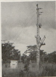
PHOTOGRAPH No. 6. Standard 11/0-38 kV. pole mounted transformer with associated equipment.
