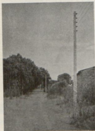
PHOTOGRAPH No. 5. Standard 38 V. overhead line construction on 28 ft. reinforced concrete poles.
