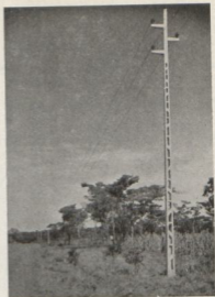
PHOTOGRAPH No. 4. Standard 11 kV. overhead line conductor on 40 ft. reinforced concrete poles.
