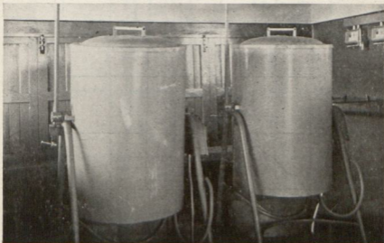
PHOTOGRAPH No. 12. 6 kW. soup boilers installed in kitchen serving meals to children in Native Township.
