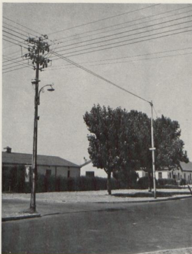
Typical construction used for overhead mains in older section of Langa Township.
