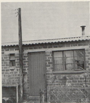
No. 6. Rear view of Married Quarters (1956) showing wooden pole and single phase incoming supply also earth to spike. This is similar to the Bachelor Quarters.
