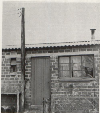
No. 6. Rear view of Married Quarters (1956) showing wooden pole and single phase incoming supply also earth to spike. This is similar to the Bachelor Quarters.
