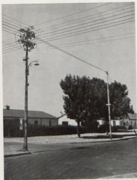
Typical construction used for overhead mains in older section of Langa Township.
