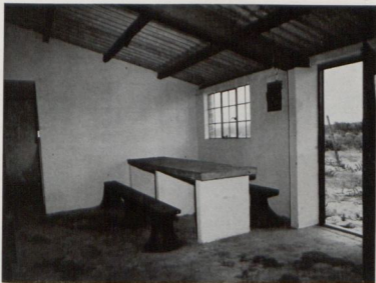
No. 9. Bachelor Hostels. View in kitchen showing position of distribution board and 4-gang switch in passage.
