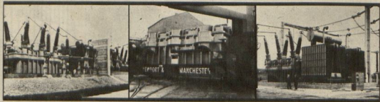
Two Parsons 500 MVA auto-transformers interconnecting the 400 kV and 275 kV grids at the Elstree sub-station, Hertfordshire.
