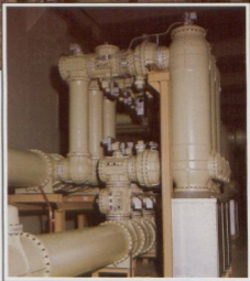
275 kV gas insulated switchgear at Escom's Croydon Substation, Johannesburg.
