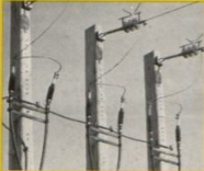
Transformers in parallel
