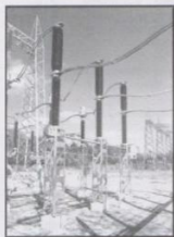
SF6 Circuit Breaker (Fig 1)
