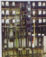
Fig. 1. Typical traditional indoor fuseboard.
