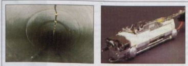
Fig. 2: An example of the BertlKomm installation robot and an example of an optical fibre cable installed in Toronto.
