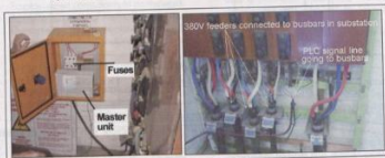
Fig. 5: Main.Net equipment connected to the electricity infrastructure
