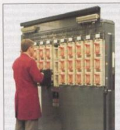
Fig. 7. Modern indoor fuseboard
