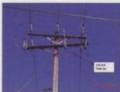
Fig. 1: "Cut-out" links were opened in order to repair a burned-off jumper conductor at Pole BB 19/B69-4 in North road, Puffontein Benoni.
