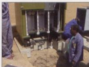
Fig. 15: Front cable access to compact switchgear.
