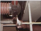
Fig. 9: Inadequate clearance due to installation of lug on 2500 A panel.
