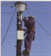
Fig. 2: Shown in the picture is a local resident who has been trained to install streetlights. Some municipalities have taken this training further and use local residents to change light bulbs thus creating work opportunities. But all electrical connections remain completed by electricians.
