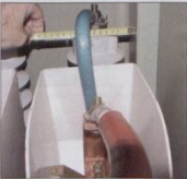
Fig. 11: Outdoor surge arresters fitted with insufficient clearances.
