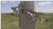
Fig. 1: Cost of repairing the damage, because of vandalism, to this high mast light was R40 000. All the luminaires, trailing cable, steel cable and the control panel were stolen. The lighting platform and door all had to be replaced due to the damage.
