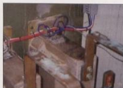
Fig. 6: Tracking on the surface (i.e. < 10 mm/kV) of a CT used in switchgear.
