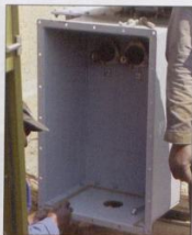
Fig. 17: CT-VT unit MV cable box.
