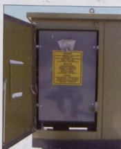
Fig. 20: Barricading of live equipment.
