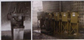
Fig. 1: – Examples of switchgear failures due to an internal arc fault in oil.
