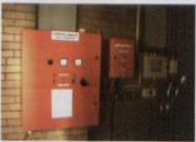
Fig. 5: CBI-electric: African Cables' 500 Hz ageing test lab and 500 Hz solid-state converter/inverter.
