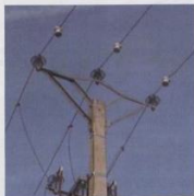
OH: Clip on fault passage indicators.
