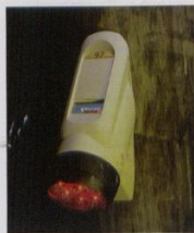
OH: Pole-mounted FPI.
