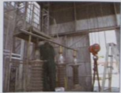
Checking the operating mechanism. A straight edge is placed on top of the three contacts to check for any discrepancies. Breaker in open position.
