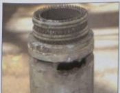
Blue phase breaking cylinder showing the melted and deformed side where tracking and arcing across to the moving contact might have occurred.
