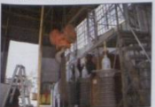
Checking the operating mechanism. A straight edge is placed on top of the three contacts to check for any discrepancies. Breaker in closed position.
