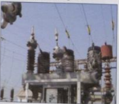
Failed circuit breaker on site.
