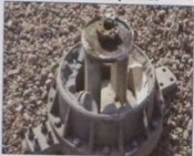
Piece of blue phase fixed arcing contact on the ground.
