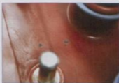
Fig. 22: Discharge from shutter box to breaker top. Discharge corresponds to the shutter hinges from the top of the breaker.
