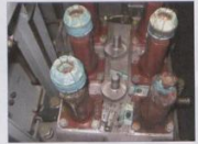
Fig. 9: Southern Sewing substation. (Note the severe degradation of insulators and cluster.)
