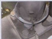
Fig. 7: Bushing failure at Junction substation.
