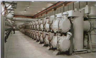
Fig. 2: GIS switchgear in an indoor substation.
