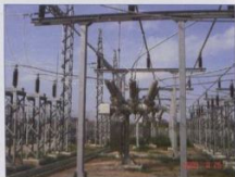
Fig. 18: PASS MOO 66 kV DBB unit used as the MTS solution in this application.
