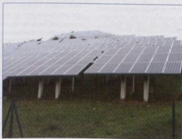
Fig. 6: Solar photovoltaic installation on old landfill site.
