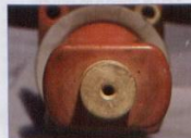
Fig. 15: Pores in Solway red phase bus bar bushing photographed at laboratory in England.
