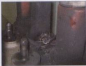
Fig. 5: Bushing failure at Santyger substation.
