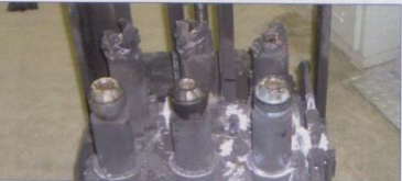
Fig. 3: Waterfront substation, Quarry breaker (Nov 05). (Note severe cluster damage.)
