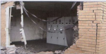
Fig. 1: Langa Metrorail substation.
