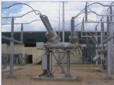
Fig. 3: Hybrid switchgear combining both AIS and GIS technologies.
