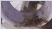
Fig. 24: Vermin guard. In many cases, degradation started between the breaker bushing and vermin guards.
