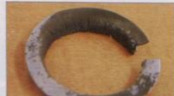
Fig. 25: Solway (short) vermin guard showing shallow depth with extensive PD tracking which eroded through the guard.
