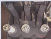
Fig. 4: Flaspack substation breaker failure.
