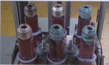
Fig. 2: Tygervalley Waterfront substation (Falls breaker) 2004. (Note the white phase bus bar side undamaged with different stages of degradation on other clusters and bushing.)
