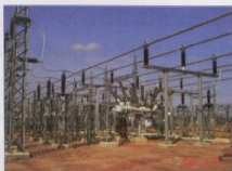
Fig. 16: PASS MO 132 kV DBB unit used as the MTS solution in this application.
