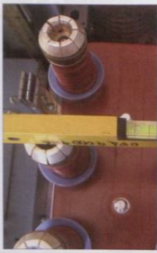
Fig. 20: Breaker supplied by manufacturer – misaligned on trolley.
