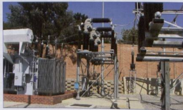
Fig. 9b: MTS transformer bay using a COMPASS unit.
