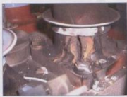
Fig. 6: Bushing failure at Faosen substation.
