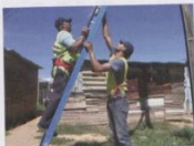
Fig. 1: Mounting a pole in the electrification project at the Langrug informal settlement.
