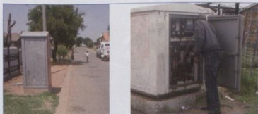
Fig. 11: Pilot Site 2 - Kerb side meter kiosks and mini-substation with RAT.
