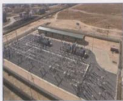
Fig. 2: A primary substation.
