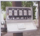
Fig. 3: Example of a clustered meter enclosure using PLC or wired split prepayment meters.
