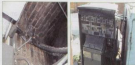
Fig. 2: The mini-substation in Bok street.
