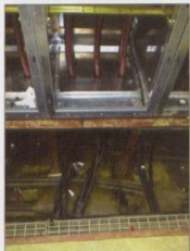
Fig. 19: Example of tri-furcating termination into compact MV switchgear.
