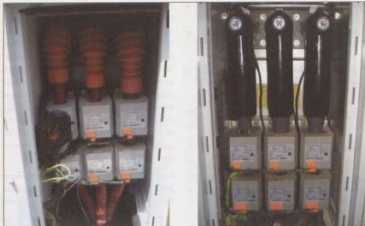
Fig. 20: Example of incorrect and correct termination into compact MV switchgear with LV CTs.
