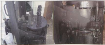
Fig. 1: Switchgear damaged in the explosion.
