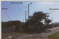
Fig. 3: Actual field photograph of equipment captured.
