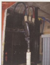
Fig. 8: Compound filled cable boxes.
