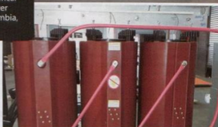
First 4MVA Cast Resin Transformers built in South Africa
