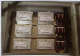
Fig. 8: Protective enclosure unit with meters inside.
