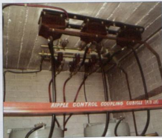
Fig. 1: Ripple control coupling cell.
