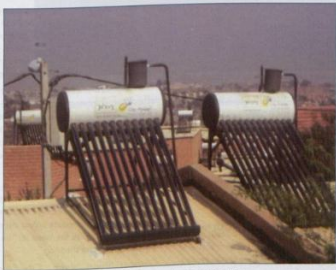
Fig. 4: Typical solar geyser installation.
