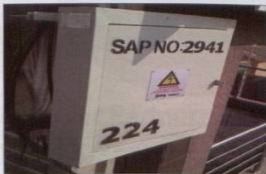
Fig. 7: Protective enclosure unit.
