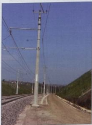
OHE masts manufactured by Aveng Infracast recently installed on the Transnet line between Bridge City and KwaMashu in KwaZulu-Natal.
