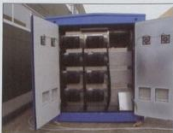
Fig. 5: Microgrid Shelter energy storage.
