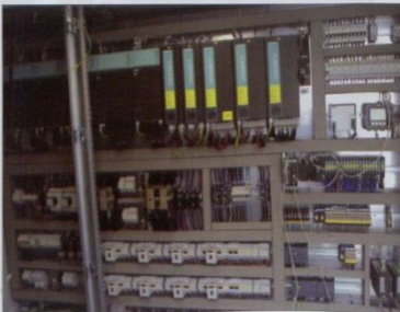
Fig. 3: Microgrid Shelter switchgear.
