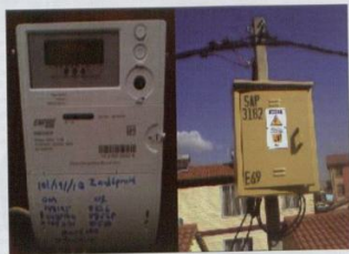
Fig. 6: Hexing meter and protective structure.
