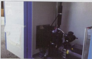
Fig. 6: Microgrid Shelter diesel generator.
