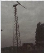
Fig. 4: Microgrid Shelter wind turbine.
