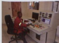
100 MVA 132 kV Testing Bay
