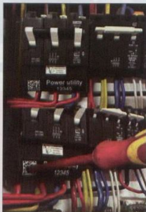
Fig. 1: Distribution board with tamper-evident labels.
