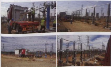
Fig. 5: CBI's EHV/HV test trailer testing 275 kV and 132 kV cable terminations at Seberaya SS.
