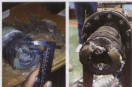
Fig. 20: XLPE insulation eroded away from the partial discharge activity. HV cable insulation will breakdown under these high electrical stresses.
