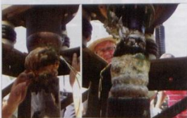
Fig. 18: Epoxy resin that is damaged due to the moisture ingress. The epoxy resin protects the main earth from moisture.
