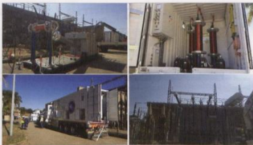
Fig. 6: MR's EHV/HV test trailer testing a 250 MVA 275/88 kV power transformer at Delta SS.
