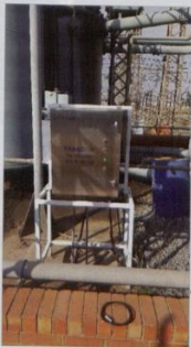
Fig. 14: Typical on-line DGA monitor installed on a power transformer.
