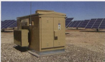
Example of an 800 kVA miniature substation installed at a solar farm.
