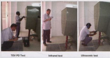
Fig. 7: Singapore technical staff performing PD testing on a transformer cable box.
