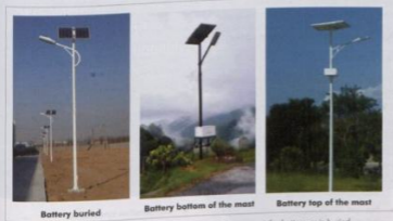
Fig. 1: The battery is placed either at the top of the mast, at the bottom or is buried.
