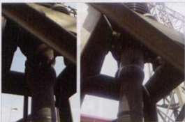
Fig. 17: Heat shrink sheath does not seal correctly and moisture enters the termination at the critical main earthing point.
