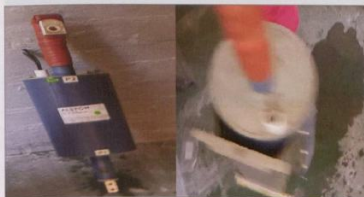
Fig. 8: Tracking CIs on 11 kV switchgear panel.
