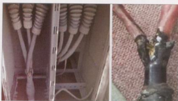
Fig. 9: 11 kV switchgear cable termination failure.
