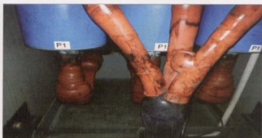
Fig. 4: Cable termination on 11 kV switchgear panel.
