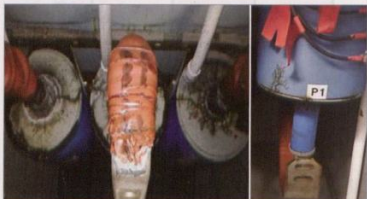
Fig. 5: Tracking CTs on 11 kV switchgear panel.
