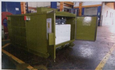
Fig. 2: Minisub with doors open, showing the RMU.
