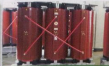
Cast Resin Transformer
