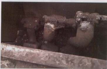
Fig. 10: 11 kV busbars failure.
