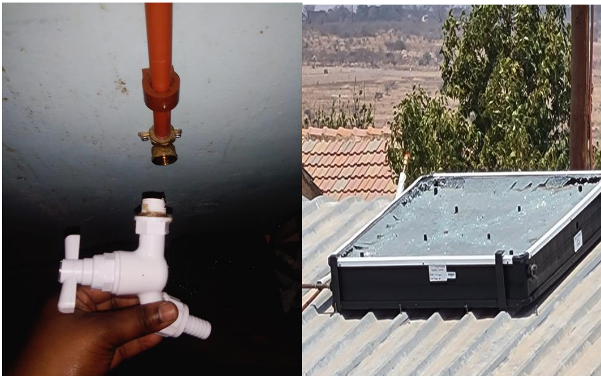
Picture of Plastic taps that overheated and went loose Geyser damaged after claiming favouritism
