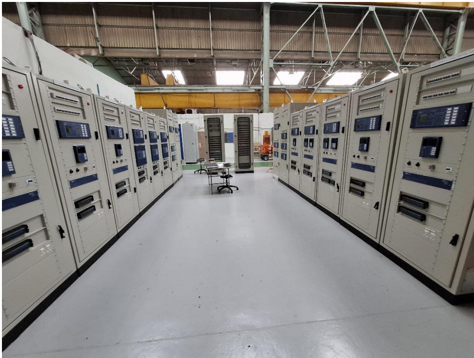
Figure 1: PAC panels ready for FAT
