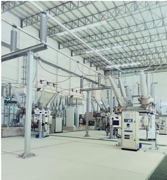
Figure 2: Compact switchgear and PAC panels in preparation for SAT
